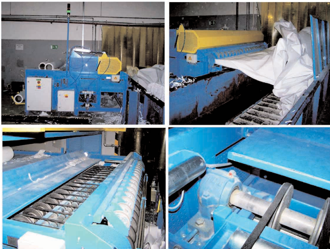
Fig. 15 Unwinding machine installed at the paperwork
