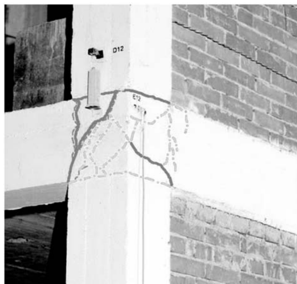
Fig. 10 Cracks in critical sections of R/C frame at the end of test - frame joint at the first floor
