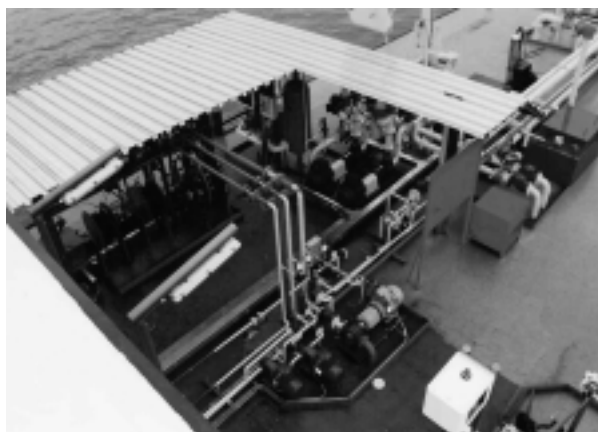
Obr. 7 Poloha čerpadiel olejov Fig. 7 Position of lubrication oil pumps
