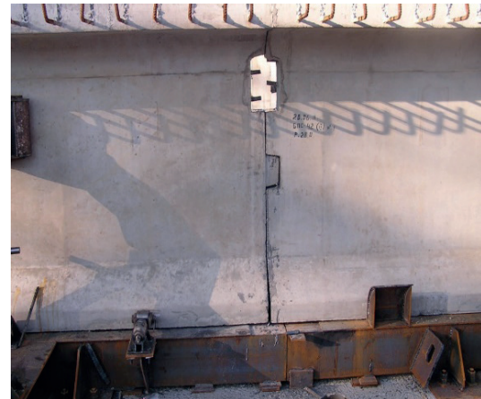
Figure 9 Missing contact of the segment heads of 42.0-m-long composite beam in No. 1 adhesive joint zone after the tension of the prestressing tendons
