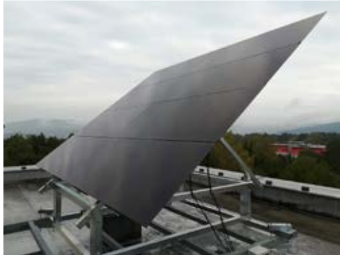
Figure 5 The PV string installation on the University Science Park's roof in Zilina, Slovakia
