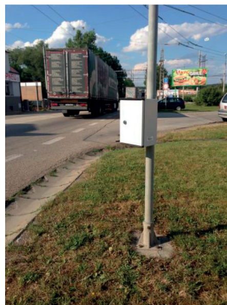
Fig. 1 Sierzega SR4 device mounted on the post of road sign - suitable for long-term measurements (source: Authors)
