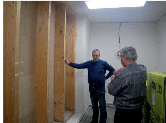
Fig. 4 Montage of thermocouples on the wooden columns from inside (November 2010)
