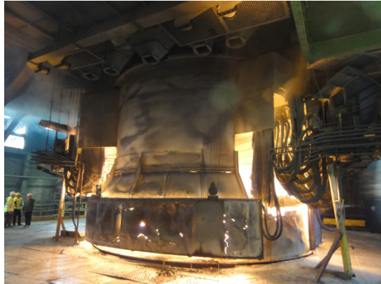
Fig. 2 ARC furnace used for ferroalloy production in OFZ, a.s. Istebne, plant Siroka
