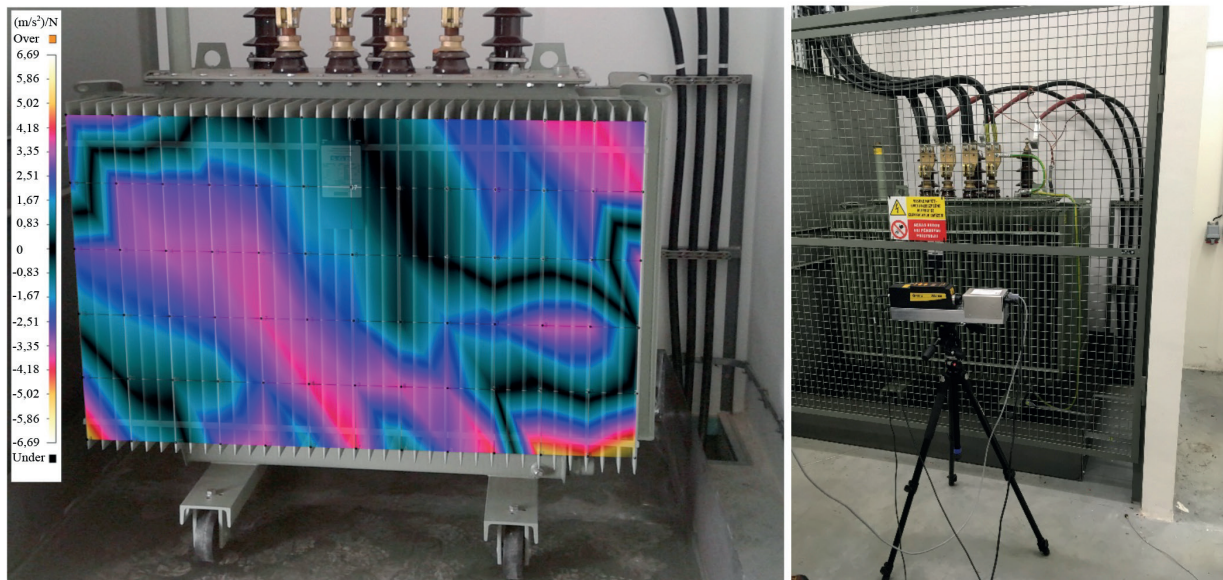
Figure 7 Measured ODS results mapped onto the transformer
