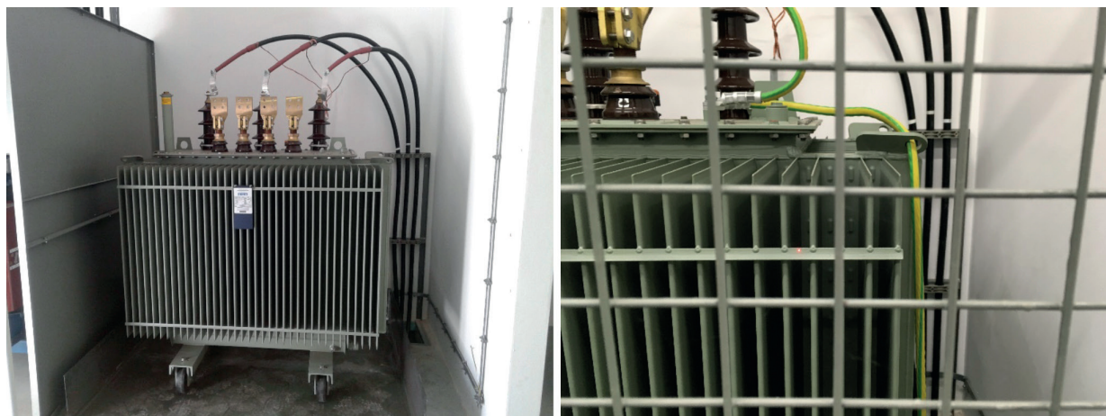
Figure 4 Tested HV transformer; without the safety barrier (left), measuring points programming (right)
