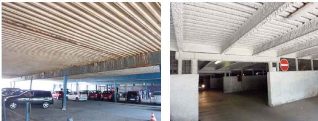
Fig. 1 The external (left) and the internal (right) roof structures of the University Hospital car park, Kosice, Trieda SNP 1
