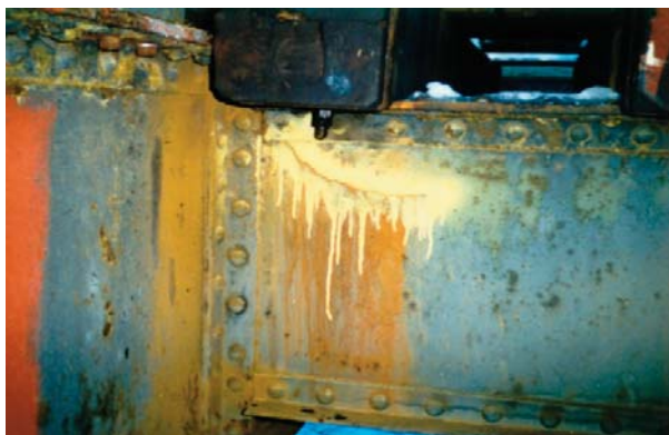
Fig. 1 Example of fatigue crack in the investigated detail
