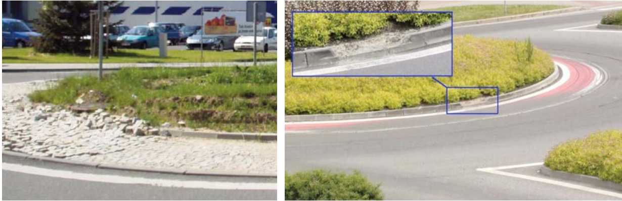
Fig. 1 Damaged truck apron and curb of the central island
