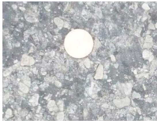
Roadway surface, asphalt concrete ACo roadway surface 11 - 15 years old (on the right)
