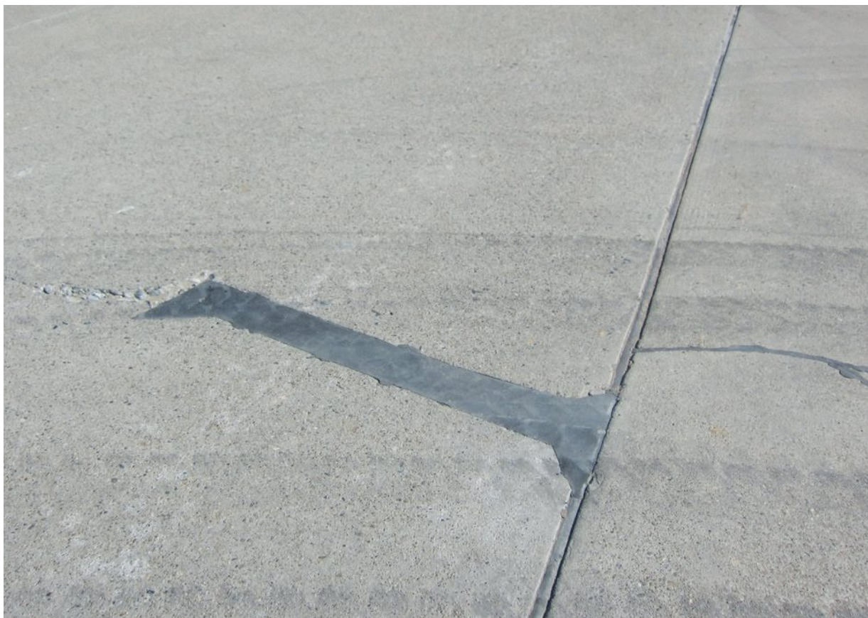
Figure 3 Intersecting cracks, cement concrete pavement slabs; author: Kazda, A.
