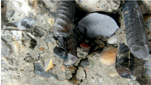
Figure 12 Detail of cut steel bars in the floor slab
