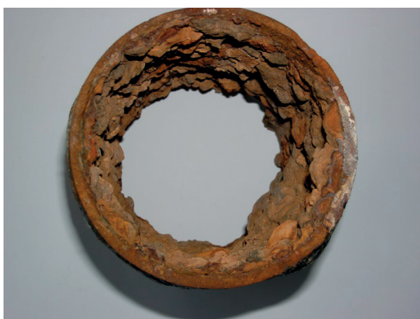
Figure 2 An example of moderately encrusted piping
