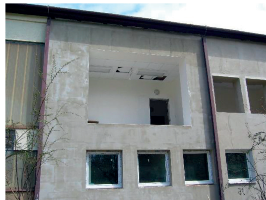
Fig. 1 Beginning of construction work on the laboratory - prepared opening for wooden frame (April 2010)
