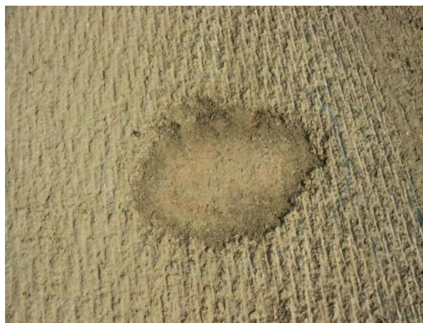
Fig. 1 Buckling under milled protective layer and surface course.
