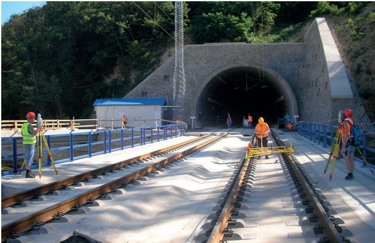
Fig. 5 View of the slab track structure of the railway bridge (diagnostics of actual and relative position of the track realized)
