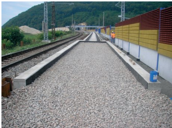
Fig. 7 View of the transition area built between the structure of the slab track and track section with standard structure of railway superstructure (left in the area of south portal and right in the area of north portal)
