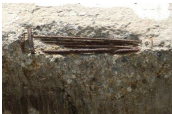
Fig. 5 The partial rupture of wires of the prestressing tendon - bridge No. 065-086
