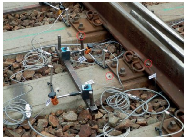
Fig. 2 Detail of a crossing part with vibration and shift sensors
