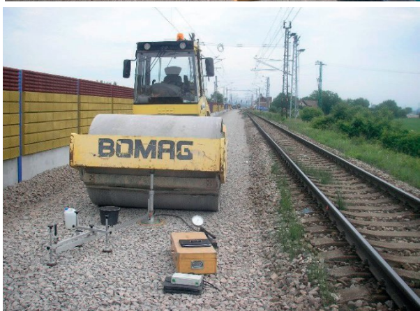
Fig. 9 Implementation of the static loading test in the northern portal (left on the surface of frost-resistant protective layer in the area of slab track, right on the surface of the railway ballast in the area with standard structure of railway superstructure)
