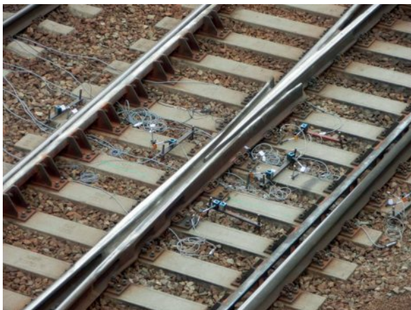
Fig. 1 General view of a frog including distributed sensors
