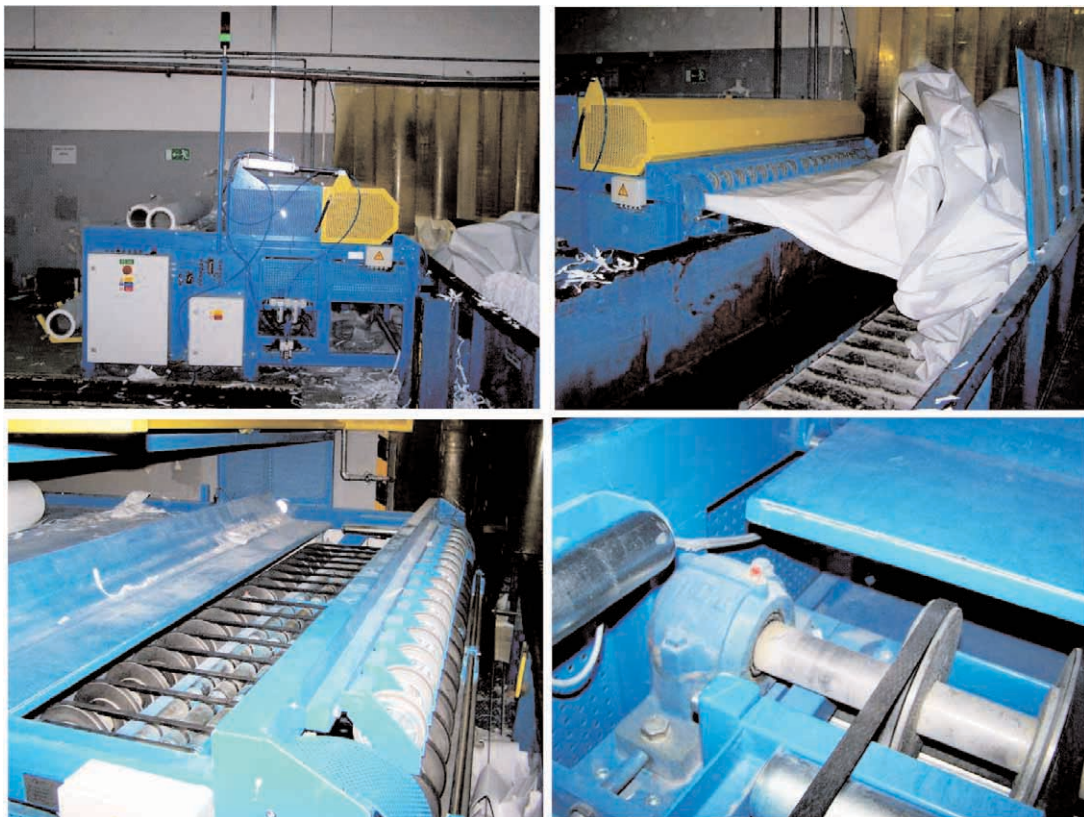
Fig. 15 Unwinding machine installed at the paperwork
