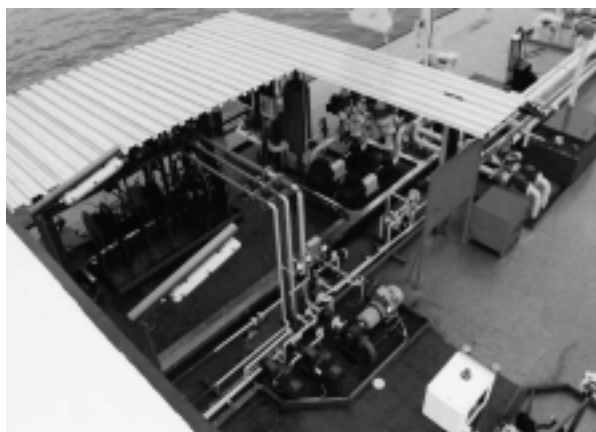
Obr. 7 Poloha čerpadiel olejov Fig. 7 Position of lubrication oil pumps
