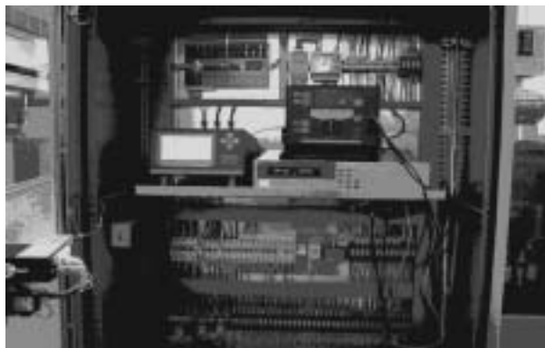
Fig. 1 The Transformer Diagnostic System
